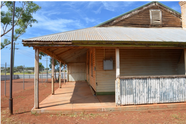
The Station Master's House shortly after work started. The yard has been cleaned up.
